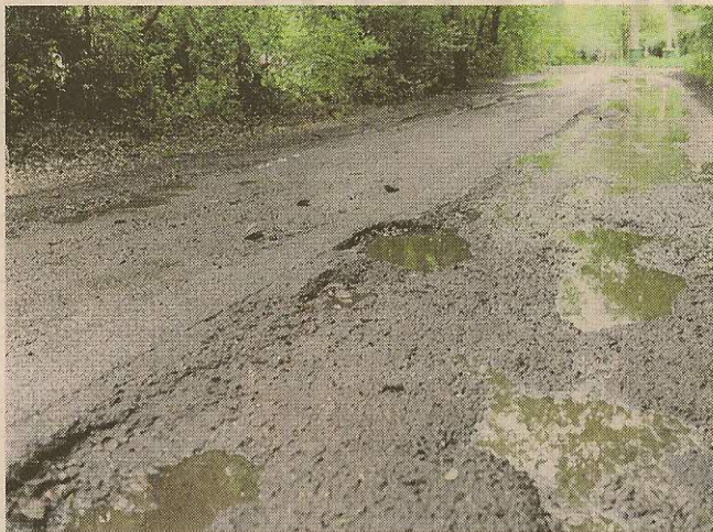
Infrastructure problems - potholes in the Horsham district
